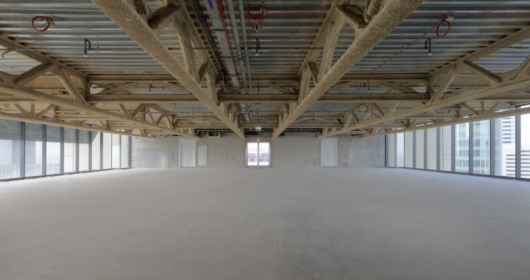
Index Tower – Shell and Core Floor (1/3 of a floor is shown here)
